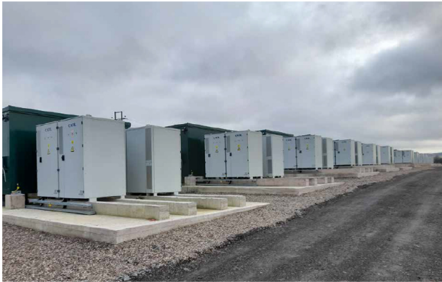
Existing battery units on site
