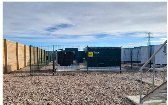
Existing battery units on site
